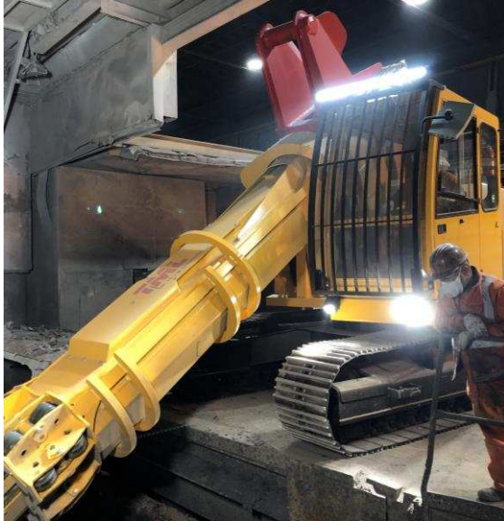
Unidachs 535 - Electric furnace outbreak
